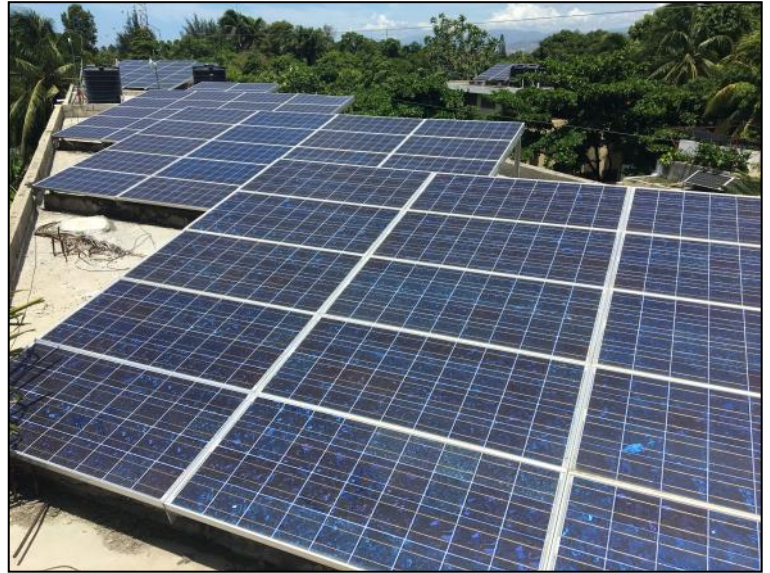
Solar panels on the Agora Building on the LCS campus, which houses the library, classrooms, and the boys' dorm. LCS's solar capabilities freed the school from unreliable utility power and drastically reduced dependence on back-up generators.
